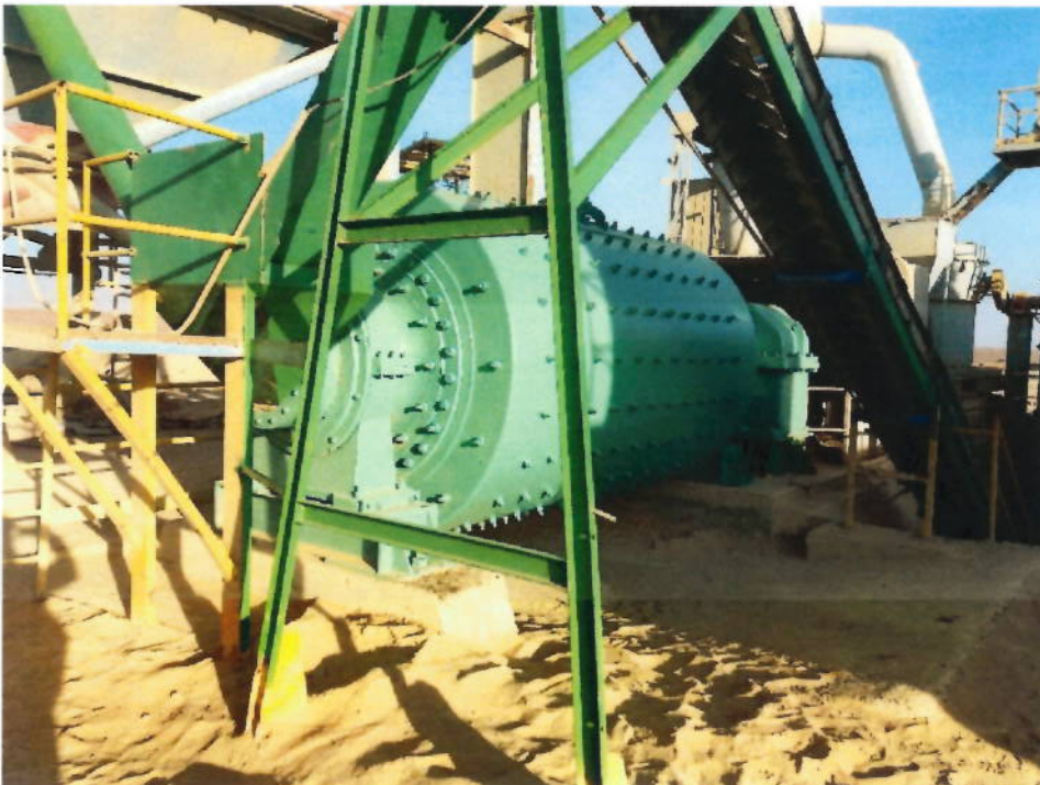
New plant installed 4 th quarter 2018
