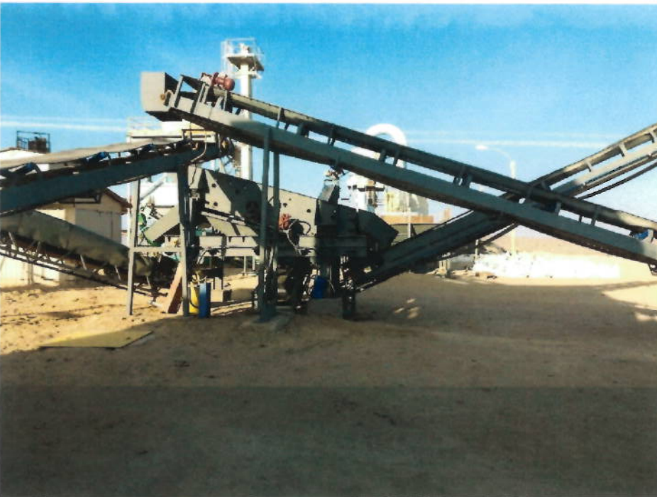
Part of new product conveyor installed 4 th quarter 2018
