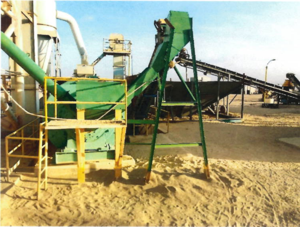
New product conveyor installed 4 th quarter 2018
