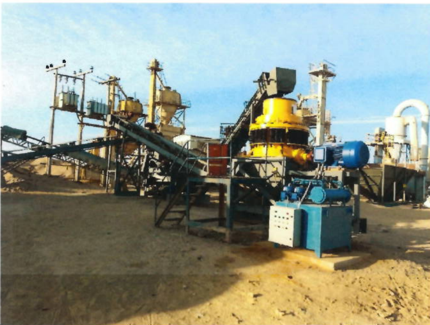
New installed plant with older equipment still utilised in background
