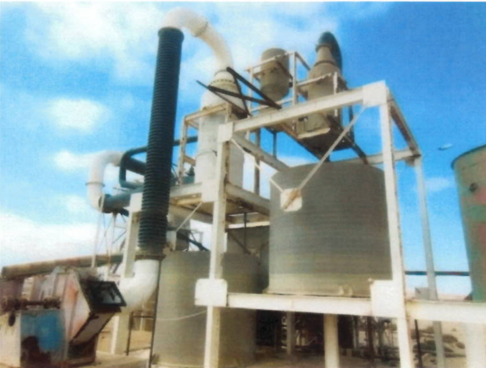
Part of on-site phosphoric acid plant
