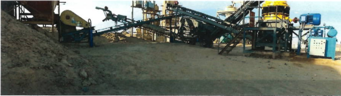
New installed plant
